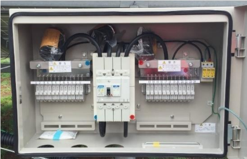
View of combiner box
