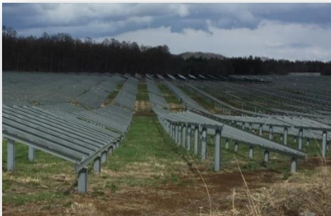
View of fix-tilt structures
