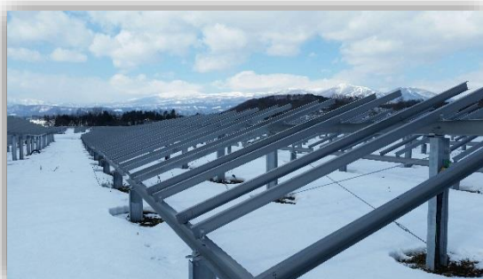
View of fix-tilt structures
