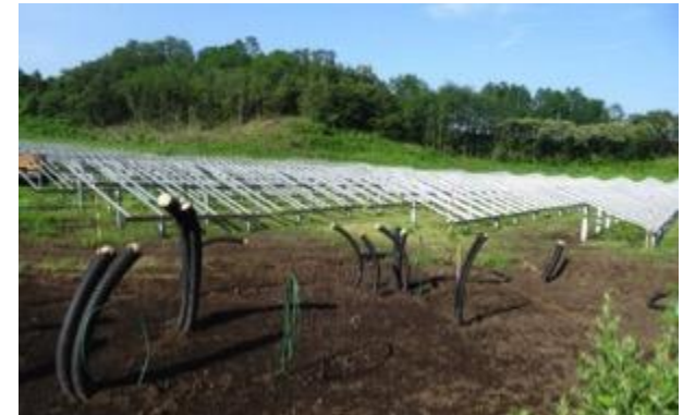
View of fix-tilt structures and DC cable conduits
