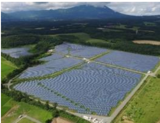
General aerial view of full plant
